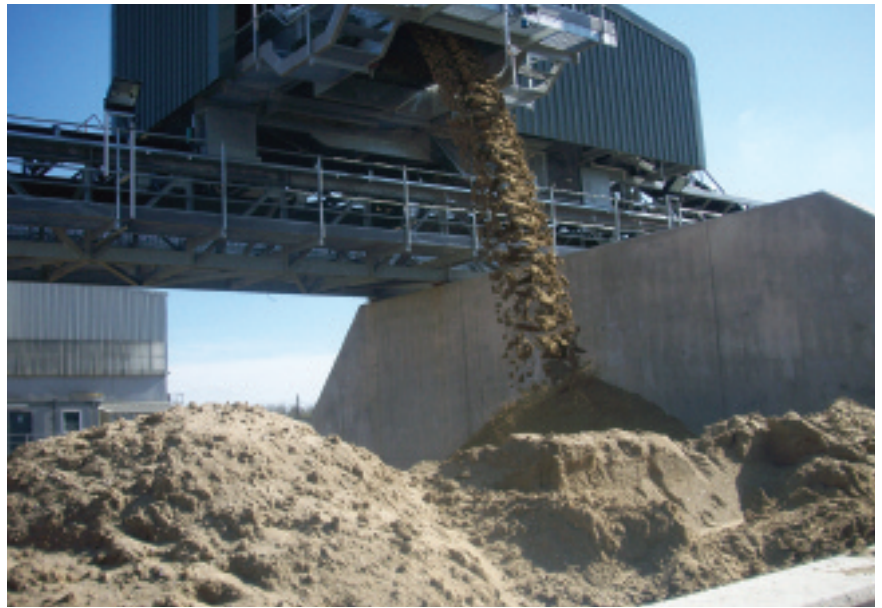
Tripper system cross conveyor discharging into one of the storage bays
