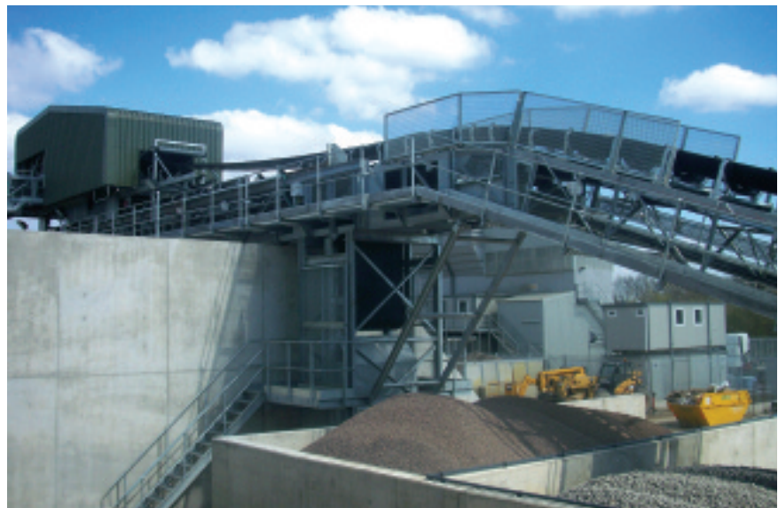
View showing the inclined feed conveyor, GTU tower and tripper carriage unit
